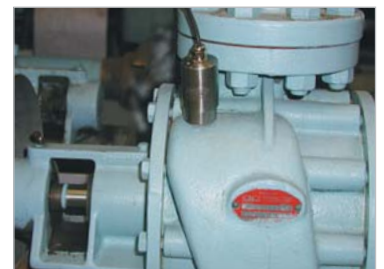
Monitor cavitation, bearings, and valves
